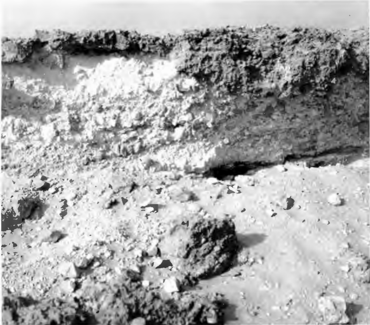
Figure 8.5. Detail of the embankment on the south side, showing the darkened weathering crust that has formed on the top of the gypsum concrete, and the horizontal division lower down between the base of the concrete and the top of the natural desert.
