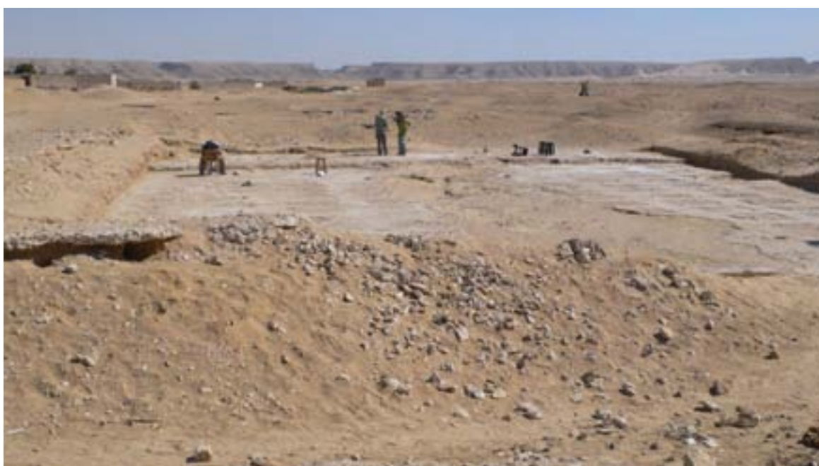
Figure 5. The gypsum concrete foundation platform at the end of the cleaning, viewed to the east.
