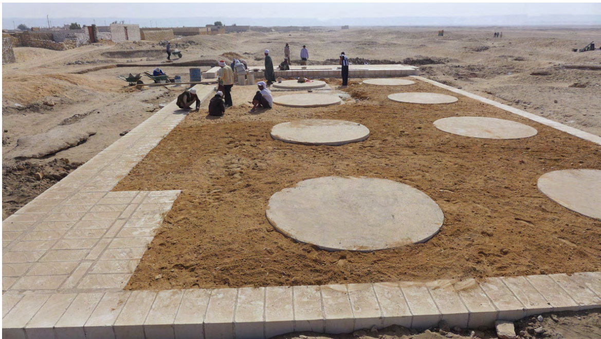
Figure 15. The final stage in the recreation of the northern pylon and its colonnade was to level up the surface with a layer of sand. View to the east.
