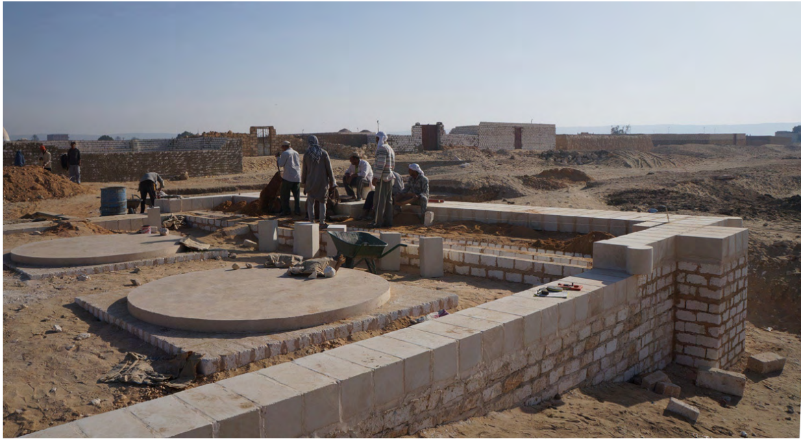
Figure 14. The recreation of the northern half of the monumental front to the temple in a late stage. The easternmost pair of the circular pads (2.5 m in dia.) which mark the positions of large column bases have been laid down. The builders are now laying the blocks of fine Tura limestone to create the shape of the pylon itself. A future stage will be to bury the foundation of small local limestone blocks completely. View to the north-east. Photo by Marsha Hill.
