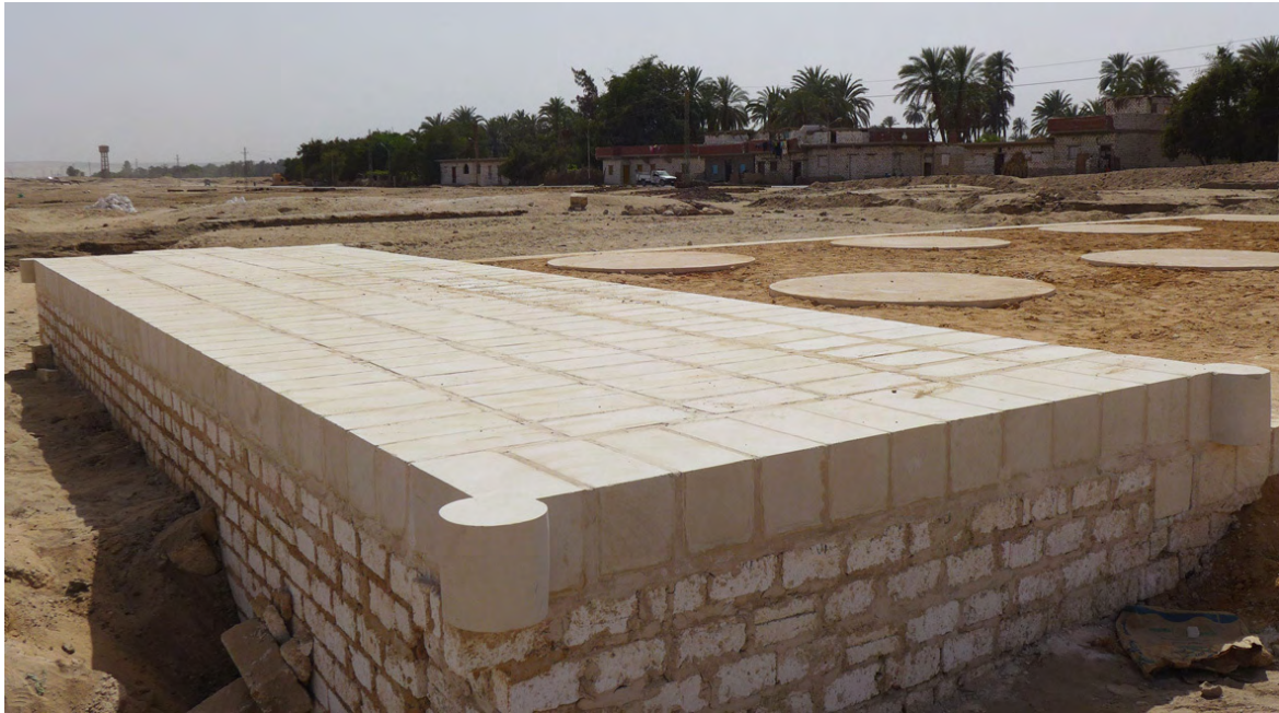
Figure 16. The north pylon as finished. The rough foundation blocks will be completely buried in the future.
