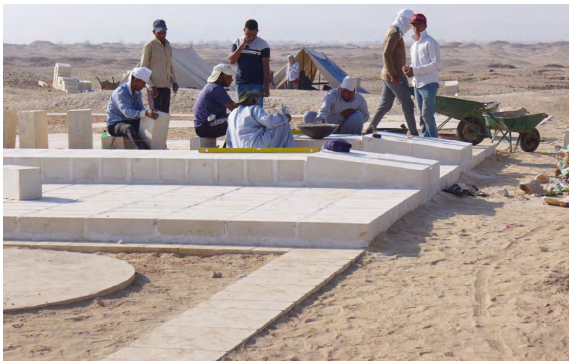
Figure 13. The building team nearing the end of the work on the front of the temple. The sloping blocks of limestone mark the start of the base for balustrade slabs which would have been inserted into the slots which have been cut down the middle of the blocks. Token pieces of red granite have yet to be inserted. View to the south. Photo by B. Kemp.
