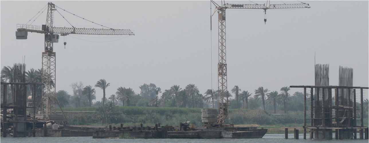
A new road bridge under construction across the Nile, linking the main west-bank highway south of Mallawi with the eastern desert near El-Bersheh. It is likely to offer direct road access to Amarna.
