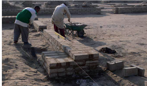
Local builder Mohammed Hussein at work, recreating the line of the front wall of the animal building.
