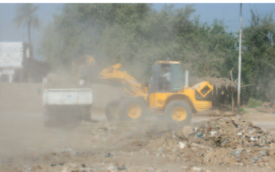
The final removal of rubbish gathered in front of the temple, carried out by the El-Till village council.
