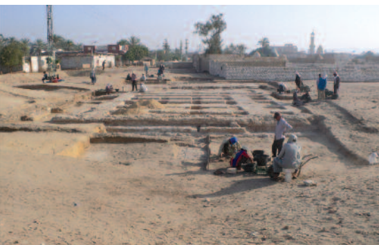
Northwards view of the excavations, with the brick pylon at the left and, occupying the centre ground, the gypsum-concrete foundations for a stone building constructed during the final phase. In the foreground the brick ramp inside the pylon threshold is beginning to appear.
