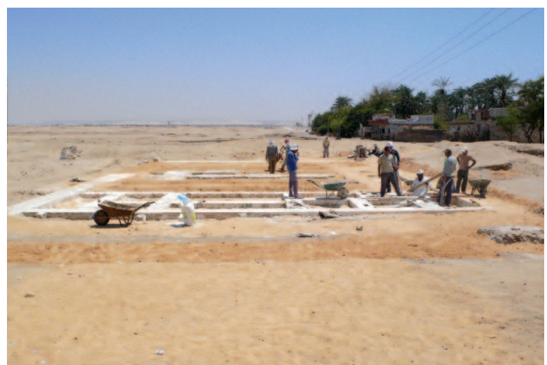
The Platform Building, viewed to the south near the end of the season. The building team from El-Till, headed by Shahata Fahmy, lays a new foundation layer of stones and mortar over a bed of sand on top of the ancient foundations. This is, in turn, covered with sand pending the completion of the work in a future season.
